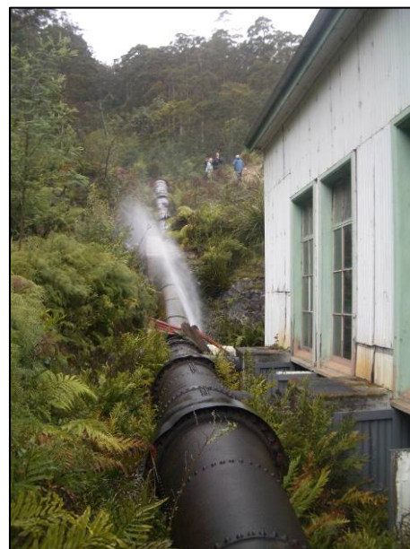
Moorina pipeline leak.
