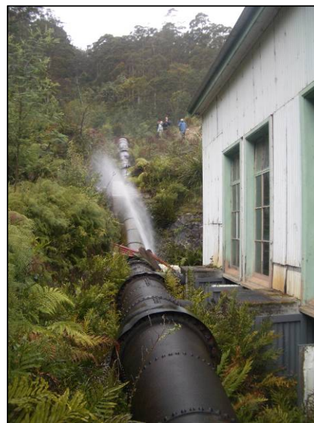
Moorina pipeline leak.
