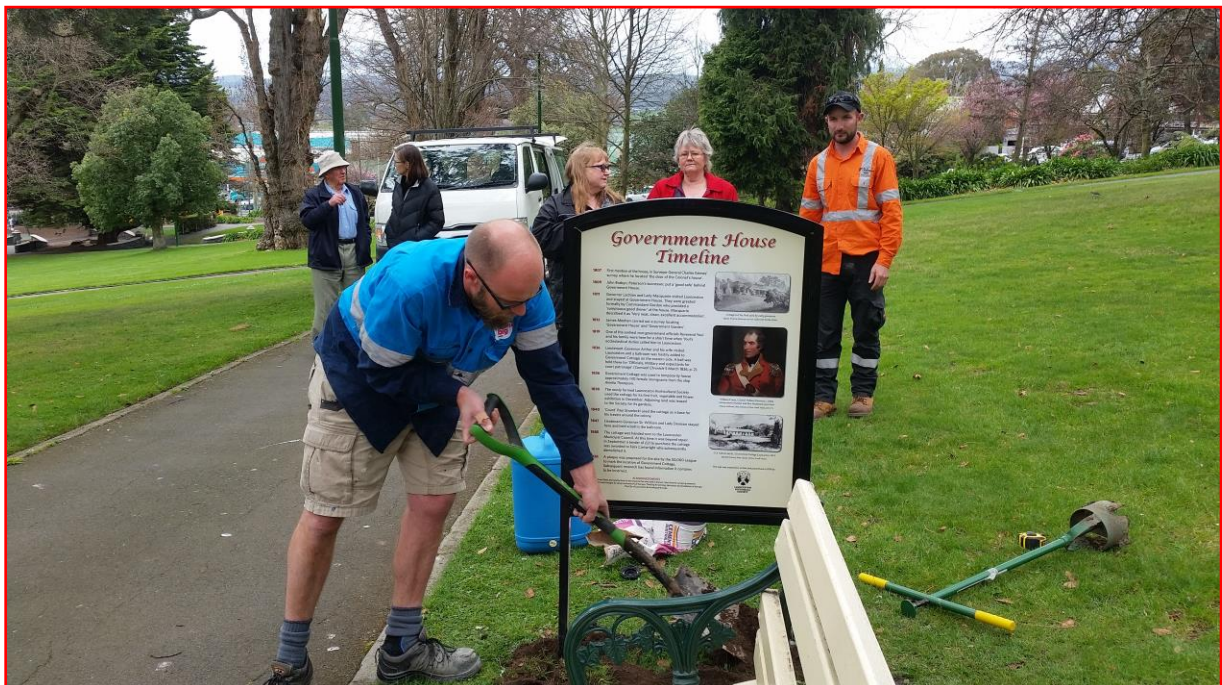
Think Big employee installing the sign in Launceston's City Park on 11 September 2018.
